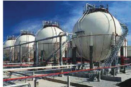
Nghi son refinery factory
